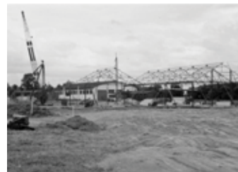
Construction of main factory buildings, with the current Goods Inwards building in the background. (Denham)
